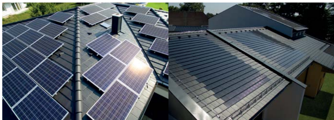
Large solar panels on top of the roof
